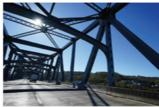
The Brent Spence Bridge - built in 1963 and maintained by the Kentucky Transportation Cabinet - transports about 160,000 vehicles a day over the Ohio River. That's twice the volume it was designed for. Photos: Spencer/The Enquirer
